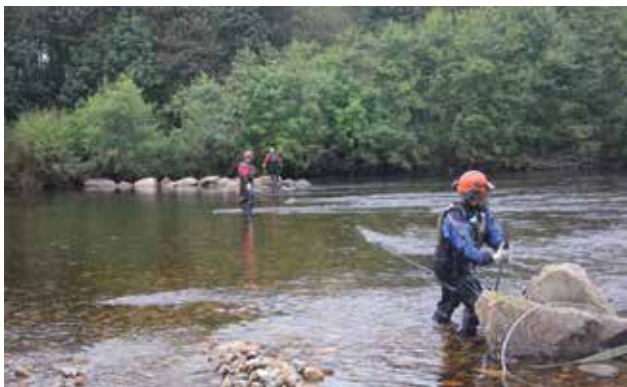
Figure 5.8 Removal of a 'croy' structure (deflector) by using hand winches on the River Dee, Aberdeenshire to restore the continuity of water flow, sediment movement and river-bed habitat (© River Dee Trust).
