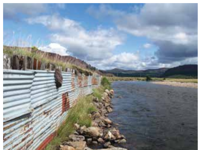
Figure 3.4 (Above) Bank reinforcement to stop natural erosion constructed from boulders on the Ewes Water, Dumfries and Galloway (© Martin Janes, RRC) and (Below) using corrugated iron and rubble on the River Dee, Aberdeenshire, Scotland. The River Dee bank reinforcement was removed in October 2015 to improve connectivity with the floodplain (© James Hutton Institute).
