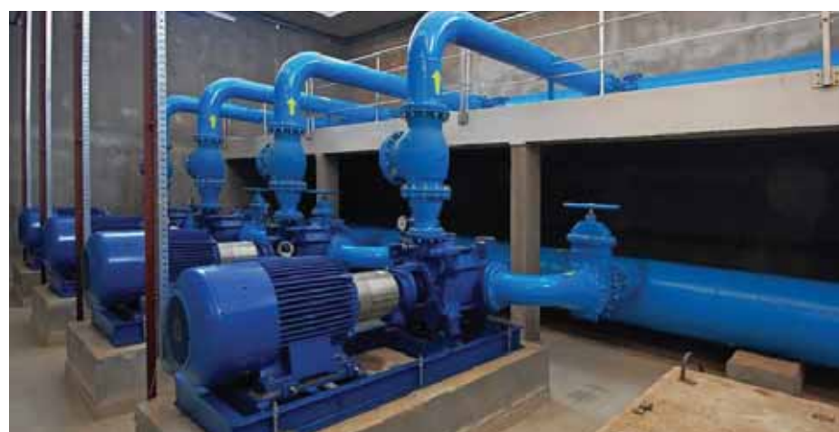
Image 16: A major pump station in a water distribution system. (Source: DMU, 2015)
