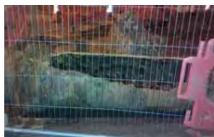
Image 12: Corroded pipe which was a source of major burst in Leicester 2015. (Source: DMU, 2015)
