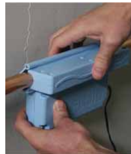
Image 19: Non-invasive 'clip-on-pipe' smart water meter. (Source: DMU, 2015)
